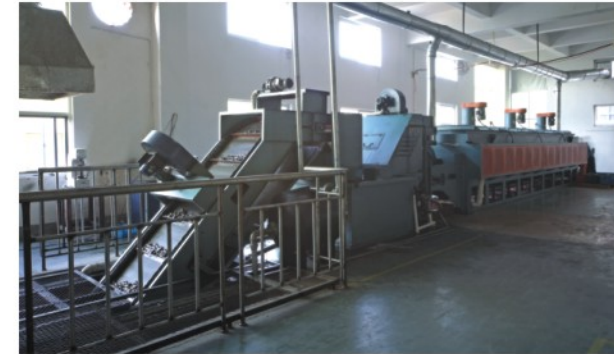
▲ 热处理设备 Heat Treatment Equipment
